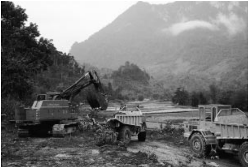
Construction of a forest road near Ham Yên, using heavy machinery from Sweden.
